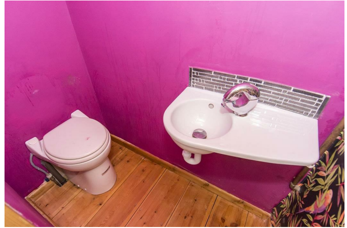
WC. Wash hand basin, Extractor fan.
